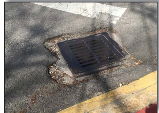
Uneven pavement concern at East Street and State Street crosswalk
