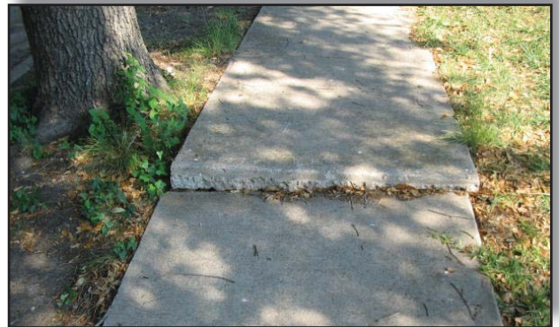
Tree Root Damage to Sidewalk Example
