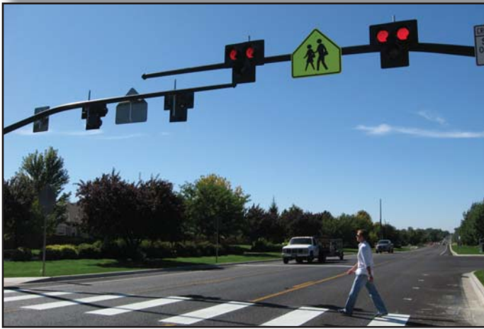
Overhead Pedestrian Crossing Signal Example
