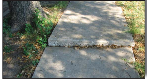
Tree Root Damage to Sidewalk Example
